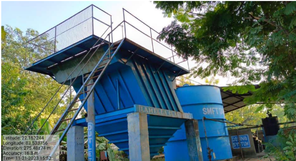
Effluent Treatment Plant # 01
