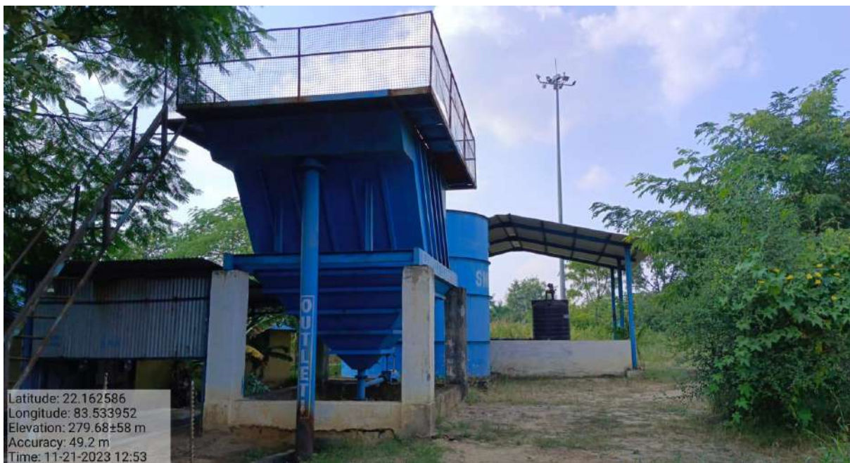
Effluent Treatment Plant # 02
