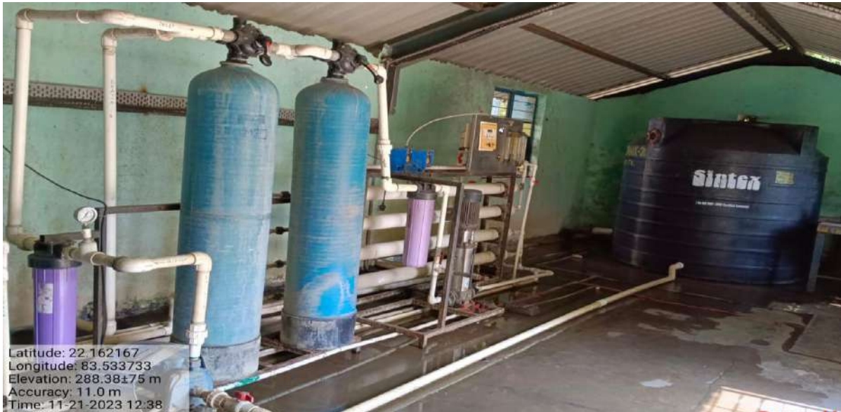
Reverse Osmosis Plant # 01
