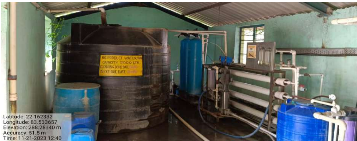
Reverse Osmosis Plant # 02
